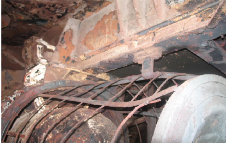
The burned horizontal sub-baskets ventilator
