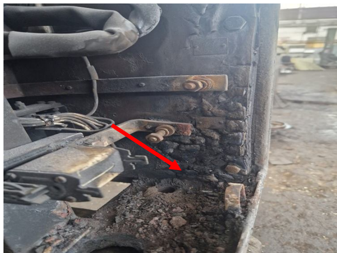
Fig. 4.11. Burnt insulation board.
