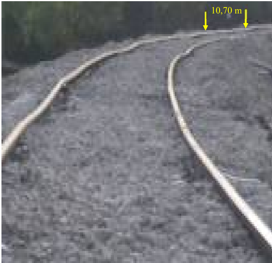
Fig. 4.15. Condition of the rail track under level at the place of derailment, measured on the basis 10,70 m of the sixth wagon
